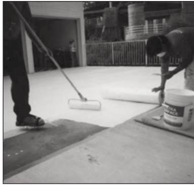
Lay the next row of fabric, so it overlaps the edge of the previous row 2-1/2 – 3". Continue laying rows of fabric until the whole surface is covered.
