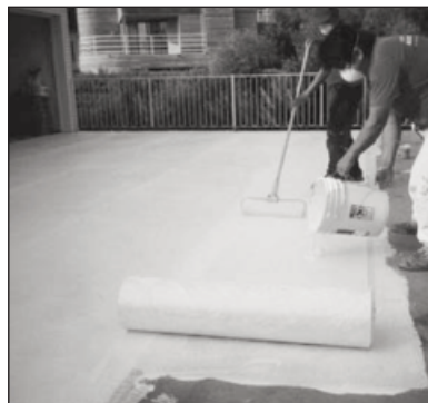
Apply Elastomeric Basecoat on top of the fabric at 100 sqft per gallon after rolling it several feet and lightly broadcast some #60 silica sand.
