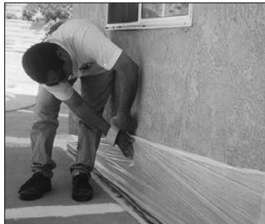
Protect surrounding areas.
