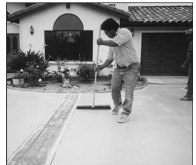
Apply a Fine Broom Finish or Swirl Pattern Finish over the dry Bond Coat (Resurfacer).
