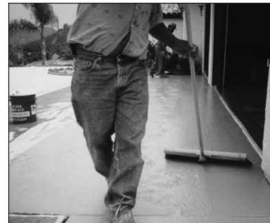
2. Spread the Fine Broom Finish material to a thin even coat next to the starting edge using a metal squeegee and broom to the desired finish.
