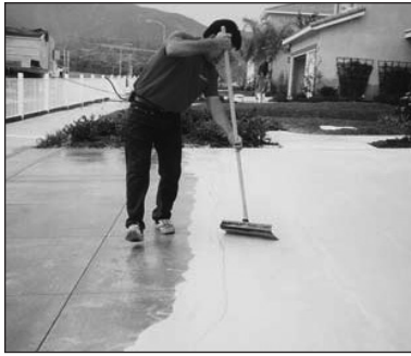
3b. Continue spreading the material ahead of the person brooming using the metal squeegee.
