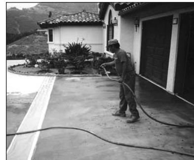
1. Make sure surrounding areas are taped off and fog the surface with water where you wish to begin spreading the material.
