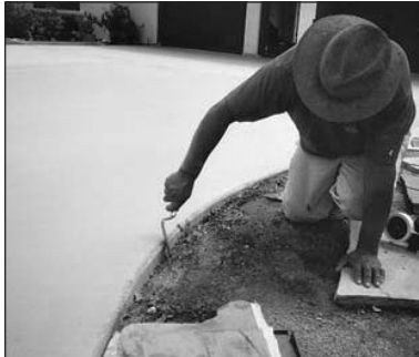
3d. Scrape or brush the vertical edges where the material drips over the sides.
