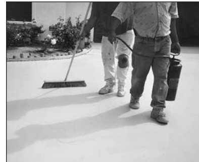
7. Apply Sealcoat 1000 using a pump up sprayer and a soft flagtip broom.
