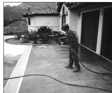
Make sure surrounding areas are taped off and fog the surface with water where you wish to begin spreading the material.
